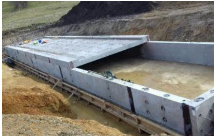
Figure 3-10: Concrete Storage System (CIRIA C753)
